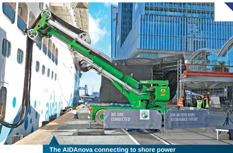
The AIDAnova connecting to shore power
